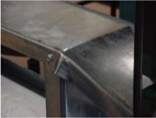
Figure 4.11-Buckling at Central Support
