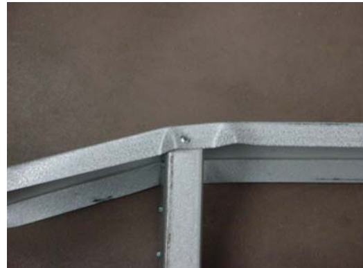
Figure 4.12-Failure of 18-ga. track
