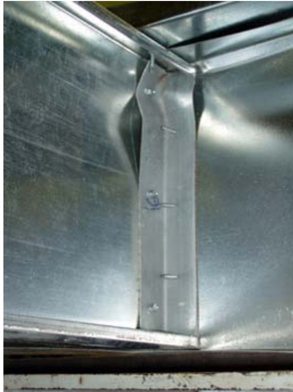
Figure 5.1: Photograph of a Clip Angle Failure
