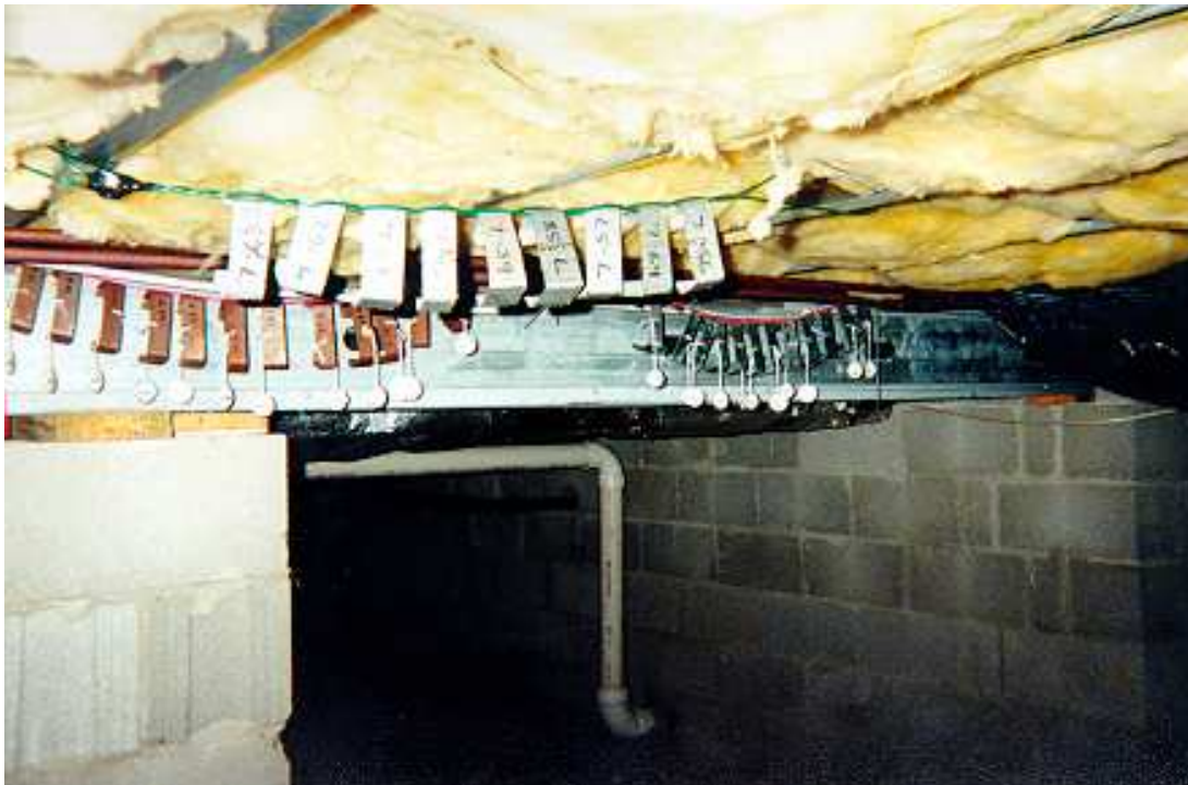
Figure 6 – Stud Specimen in Leonardtown Site Crawlspace
