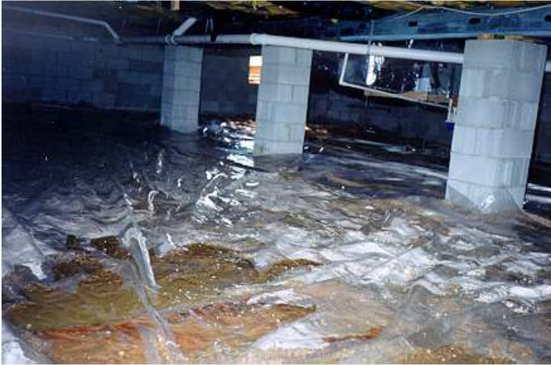
Figure 7 – Water (Foreground) in Leonardtown Crawlspace
